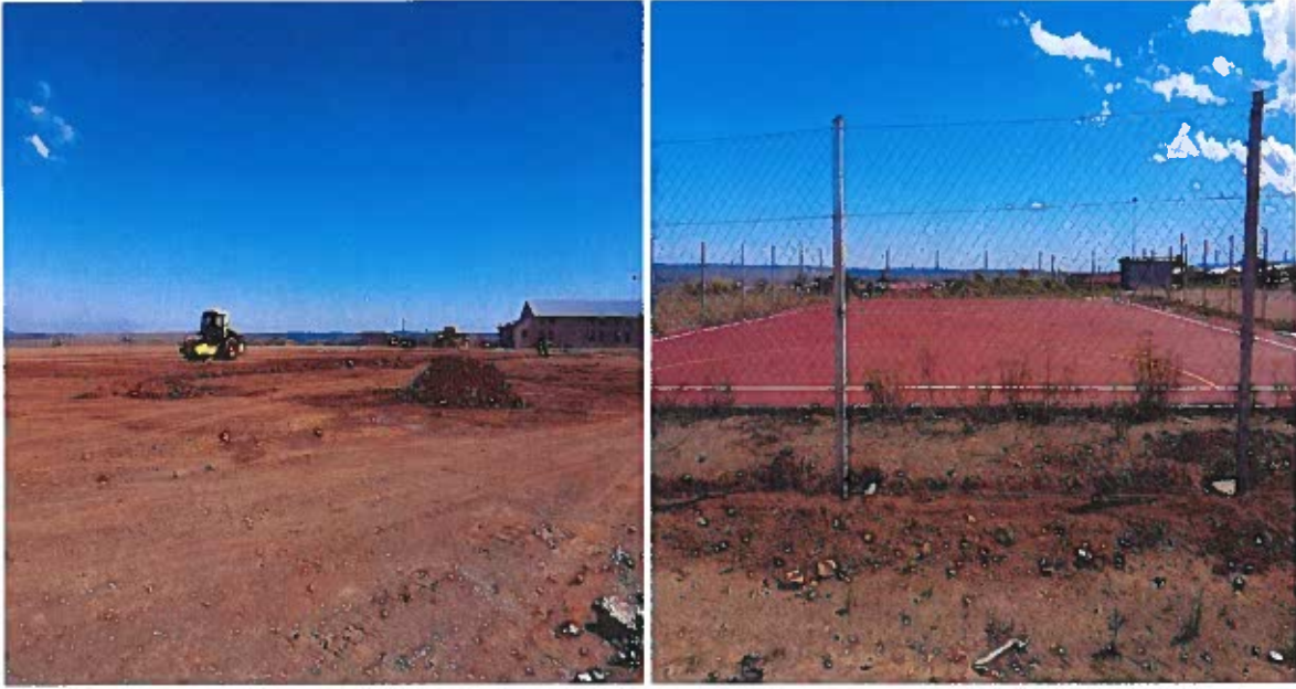
The contractor was terminated in June 2023 and the scope for tender to finish the work is being finalized.
